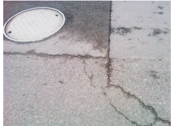
Square cut repairs routinely develop extruding cracks. Whereas circular cut repairs typically maintain solidity.
