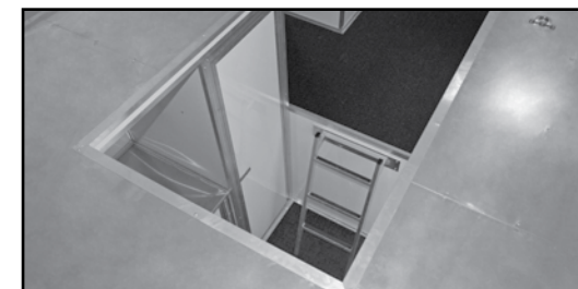
Notch in Platform with Angled Removable Ladder from Main Floor to Bunk at Riser
