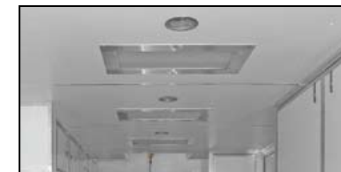
Recessed Thinline Fluorescent Lights in Platform with Recessed Dome Lights
