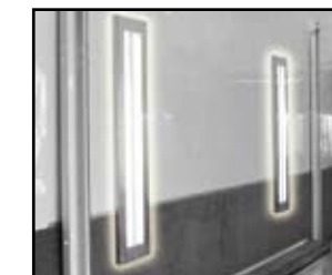
Thinline Fluorescent Lights Recessed in Interior Sidewalls
